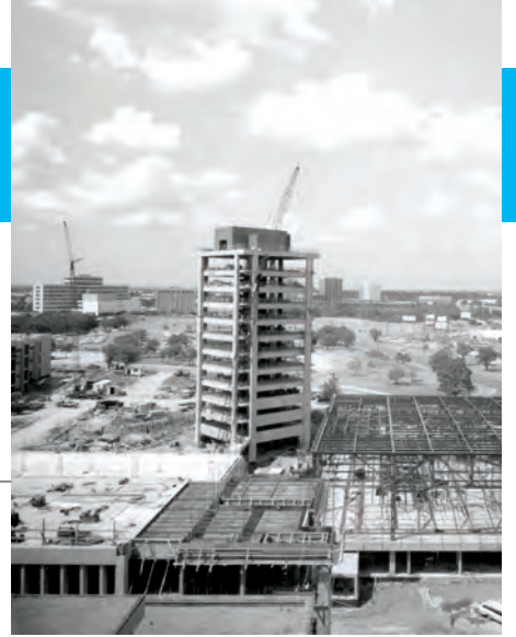
This photo, taken from the roof of the Edward H. Cary Building, shows the Eugene McDermott Academic Administration Building and the steel skeleton of the Tom and Lula Gooch Auditorium to the right. In the foreground, the Fred F. Florence Bioinformation Center building rises in front of the Cary Building.
